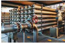
Edward C. Little Water Recycling Facility El Segundo, CA 30-40 MGD
